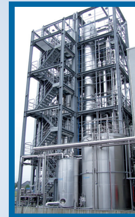
Industrial scale evaporator at Novasep Mourenx site (France)
